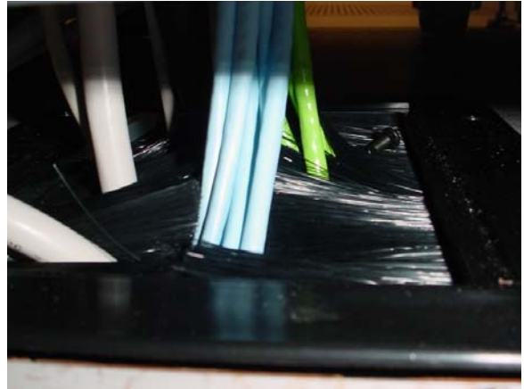
Figure 65: Brush Grommet Seals Access Floor Tile Cutout Under Equipment Cabinet
