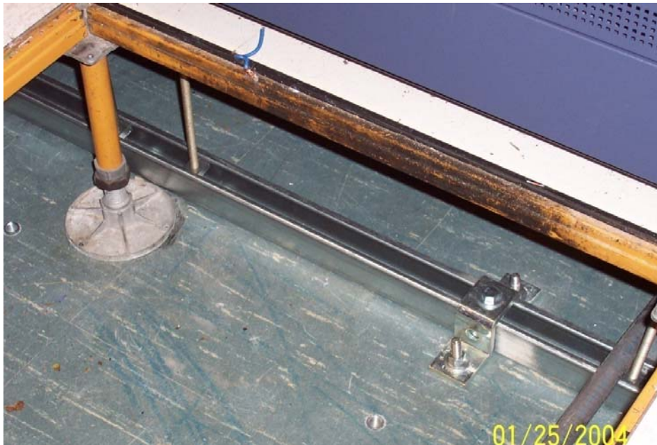
Figure 67: Method For Securing Racks And Cabinets On An Access Floor Using Threaded Rod Connected To Steel Channel Bolted To Concrete Slab
