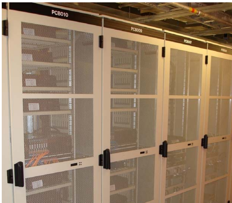
Figure 60: Cabinets Are Identified And Labeled
