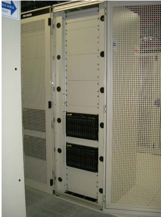
Figure 58: Blank Panels Installed In Empty RUs
